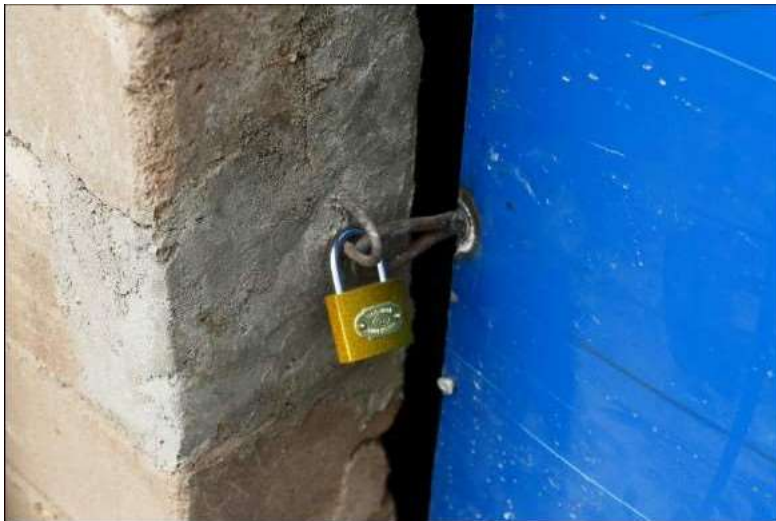
Figure 32: each door is provided with a lock, in order to don't allow external people during night/school closure.
