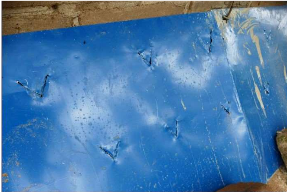
Figure 29: on the chamber sheet covered they were made some holes; in this way, the metallic sheet has no/low value, it is very less attractive at the black market and the risk of theft is much minimized.
