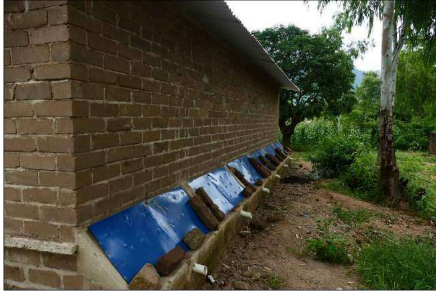
Figure 28: chamber side of a line of 6 toilets in a primary school in Phalombe District
