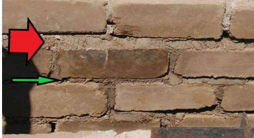
Figure 18: SSB bricks lined in an internal part of a toilet chamber. The red arrow represent the wrong amount of mortar, corresponding to about 3 cm; the green arrow represent the correct amount of mortar, about 1 cm.
