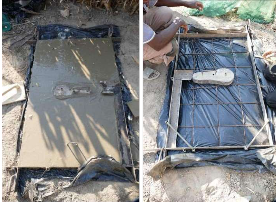
Figure 15: slab casting phase, using the mould complete with urine channel and movable hole mould
