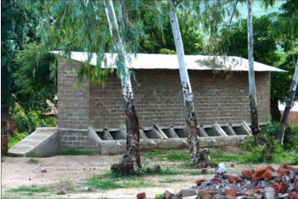
Figure 26: six ecosan toilettes built in a line, under construction in a primary school.
