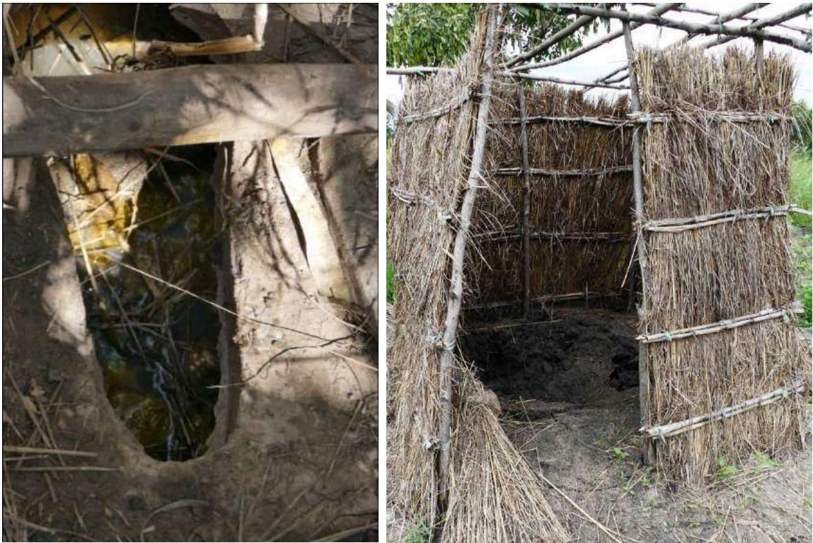
Figure 3: on the left, the pit of a traditional latrine provided with an IA concrete slab is full of sludge and rain water coming from the surface and the water table, after 2 days of rain; on the right, a temporary toilet has a collapsed pit, due to 2 days of rain, use of temporary material and absence of roofing.
