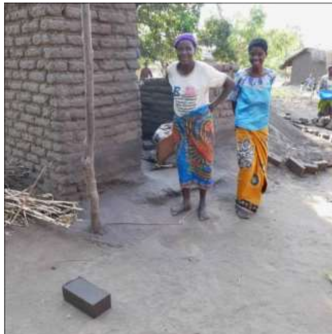
Figure 8: the very first block made in the first pilot village by the family of the lady in the picture, sanitation Phalombe program 2019-2020
