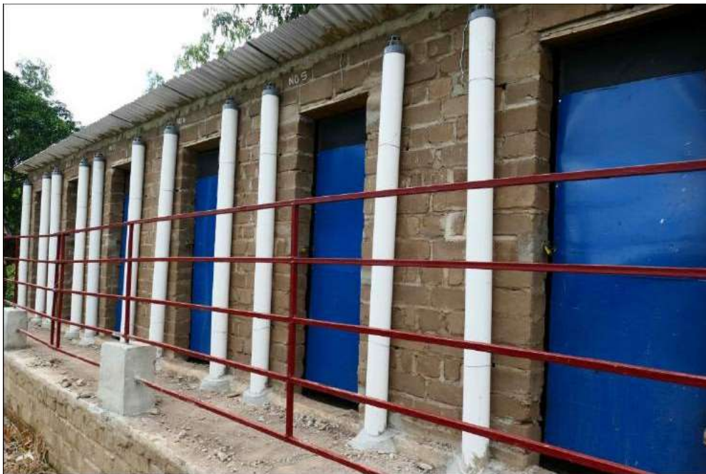
Figure 27: door side of a line of 6 ecosan toilets in working progress for a primary school in Phalombe District
