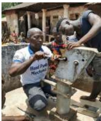
Maintenance of a Hand Pump by a Pump Technician, Bombali, Sierra Leone, 2022
