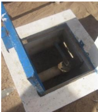
Figure 75 : Vanne de distribution
