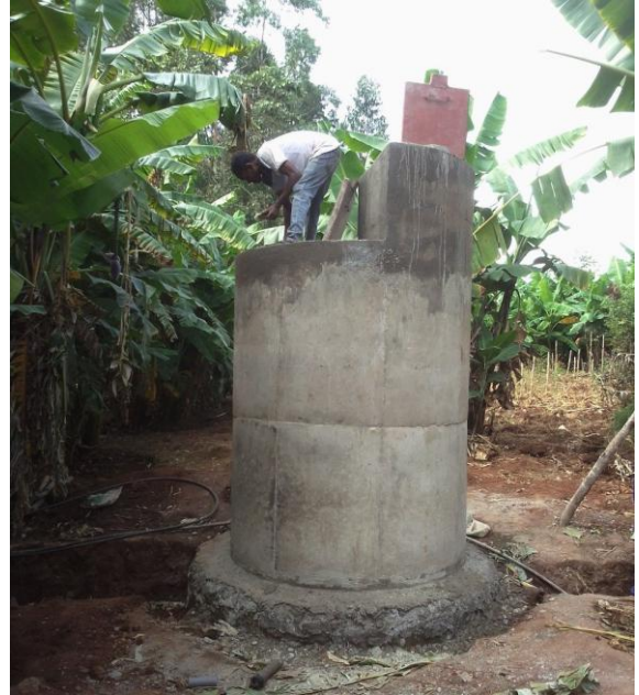
A distribution box built on top of the reservoir: one structure instead of two, close to the people who use it.
